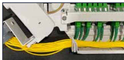
Patchcords guided to the side, protected by front door with label for port identification
